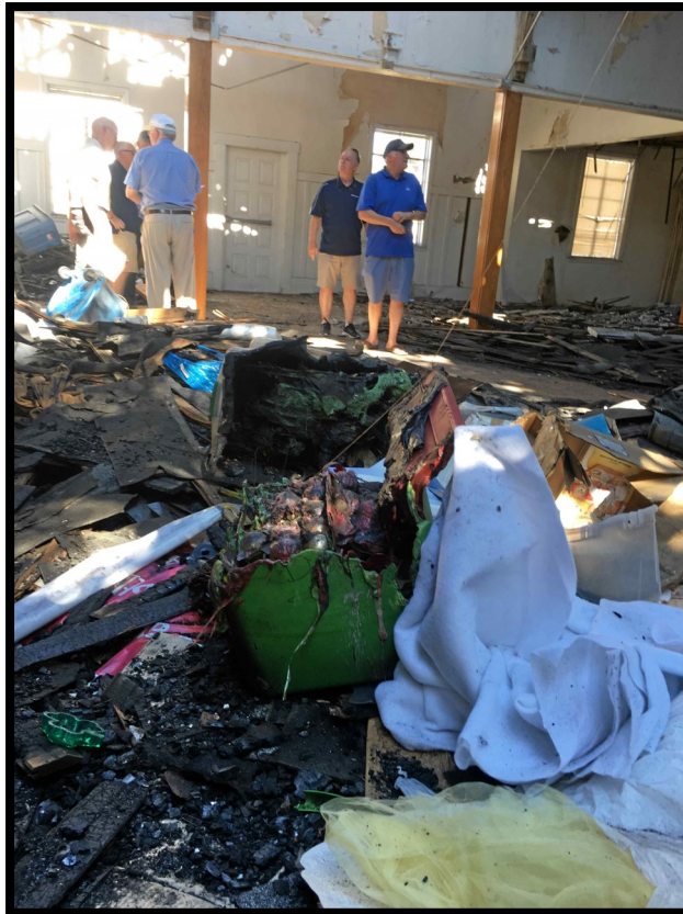
A group of city officials and local builders, developers and insurers met with members of the Reville Lions Club on Monday inside the burned out Lions Club-
